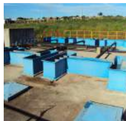
Foto: Reator UASB (biodigestor)
