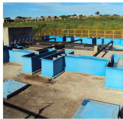
Foto: Reator UASB (biodigestor)
